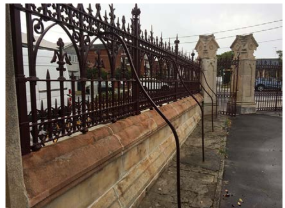
RESTORED CAST IRON BOUNDARY FENCING AND SANDSTONE PLINTH AND PIERS AT THE ENTRY
